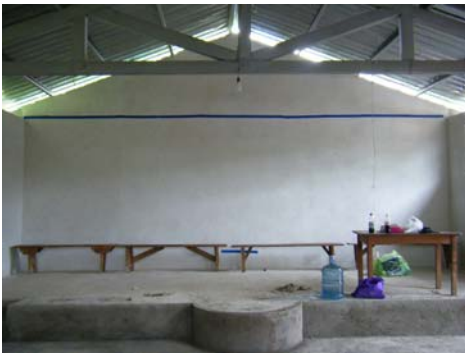
THE CHURCH WALL... "BEFORE"
