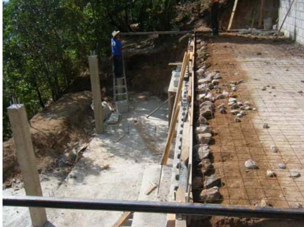
Amilio, from San Antonio, helping set up the form for the upper floor.
